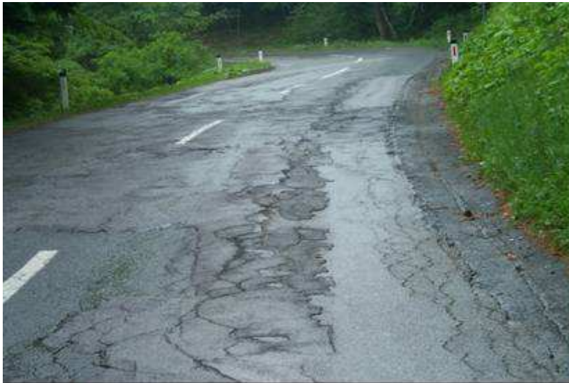
Picture 9 Pavement condition, case study No 2
