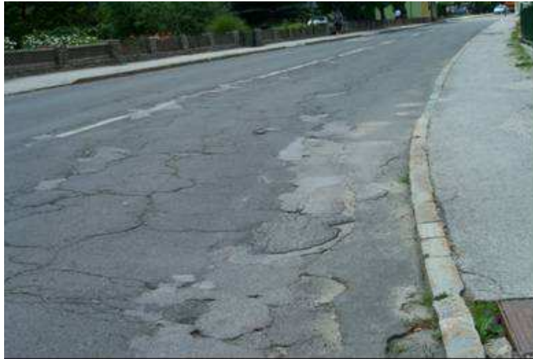
Picture 7 Pavement needing reconstruction
