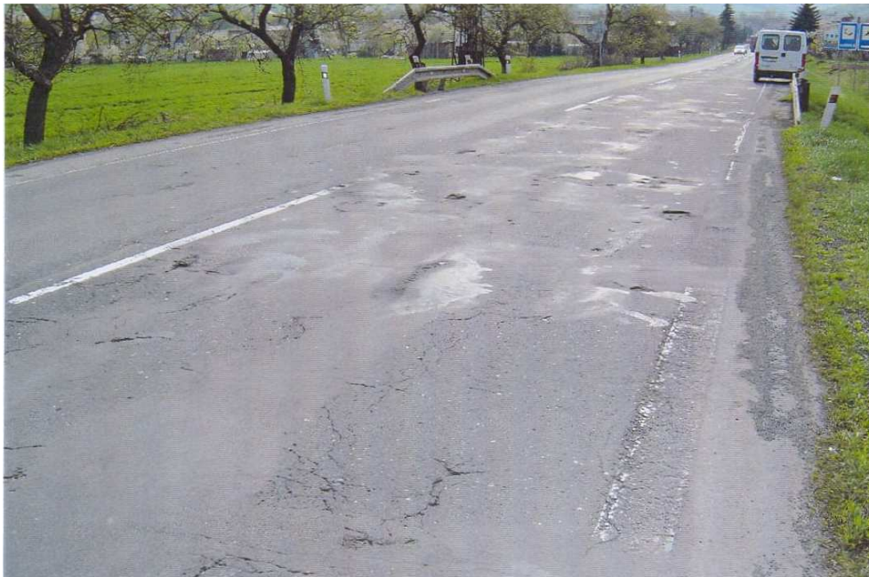
Picture 12 Pavement condition, case study No 5
