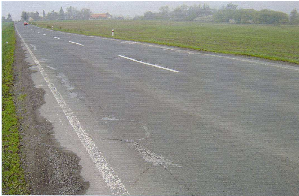
Picture 11 Pavement condition, case study No 4
