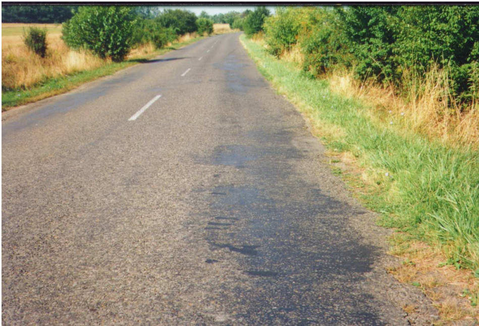
Picture 10 Pavement condition, case study No 3
