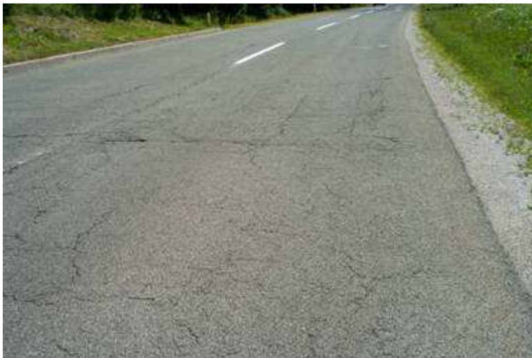
Picture 8 Pavement condition, case study No 1
